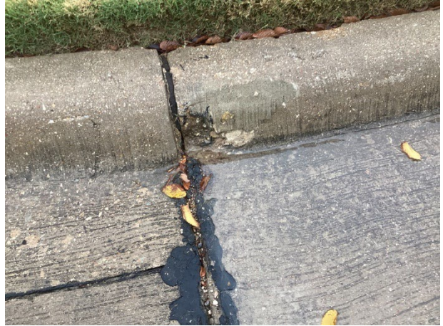
Concrete curb spalls
