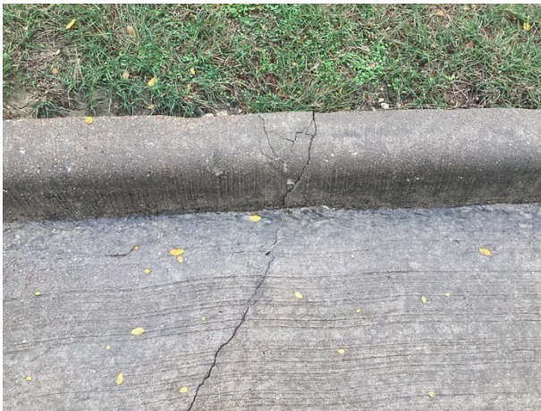
Concrete curb cracks
