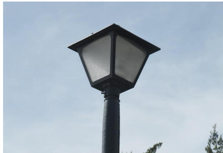
Typical fixture at light pole.
