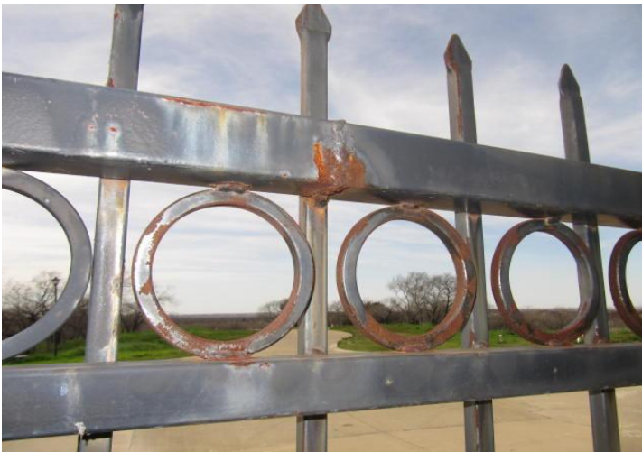
Area of poor paint finishes at metal gate.
