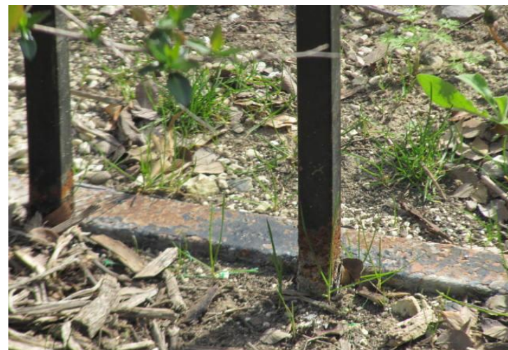
Poor paint finishes near grade.
