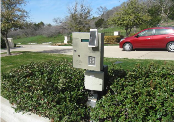
Overview of intercom entry panel.
