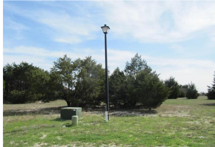
Typical light pole and fixture.
