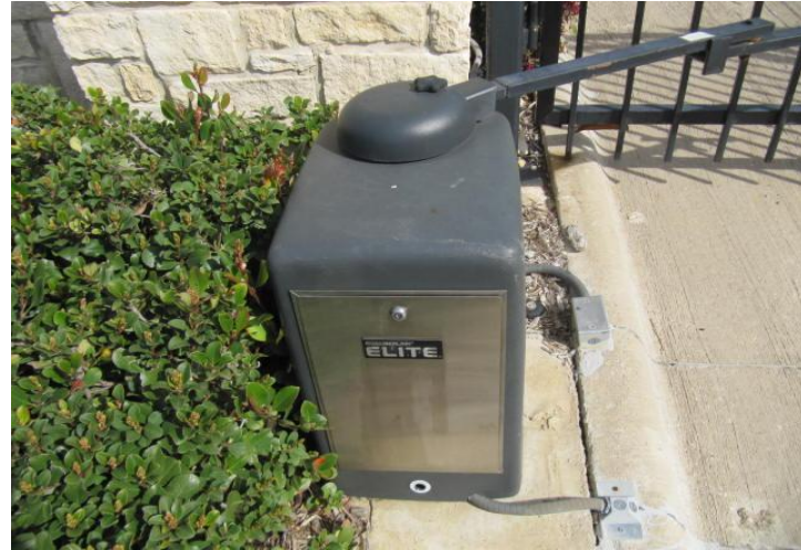
Gate operator at front entrance gate.
