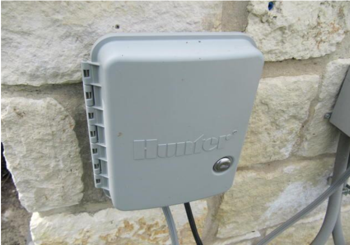
Irrigation control box.
