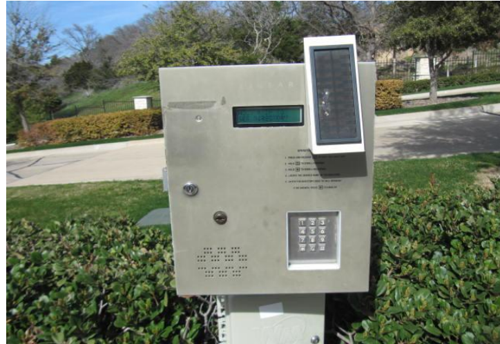
Intercom entry system with solar panel.
