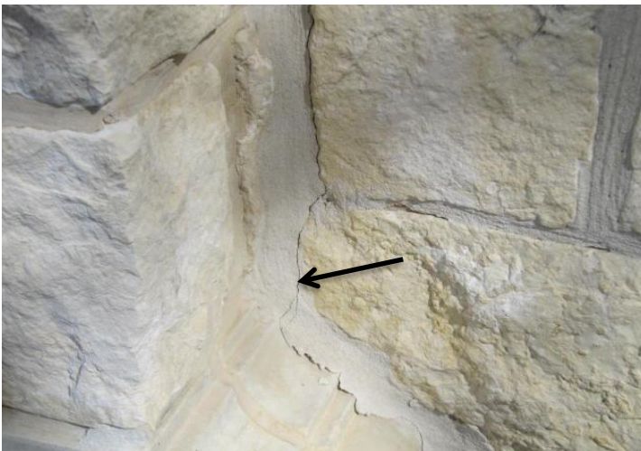
Small hairline crack at mortar joint.
