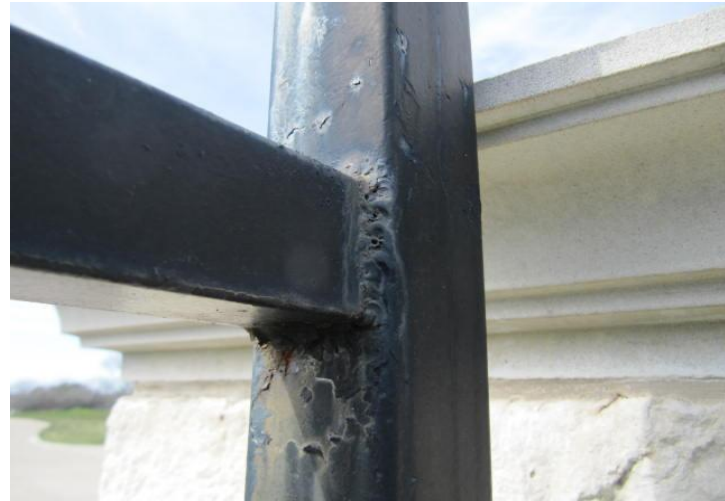
Area of poor paint finishes at metal fence post.
