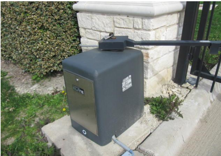
Operator for gate at rear property entrance.
